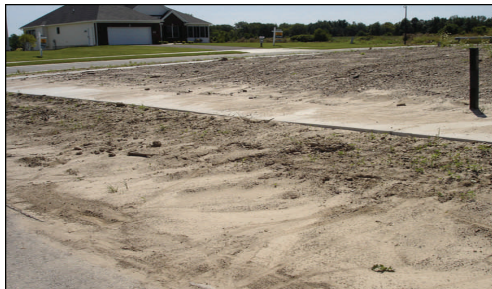
Unstabilized Construction Site.
