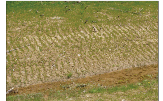
Tracking in the wrong direction leads to the formation of rills.
