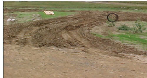
Improper construction site entrance.
