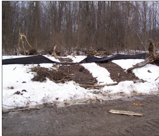
Silt fence that has been driven over.
